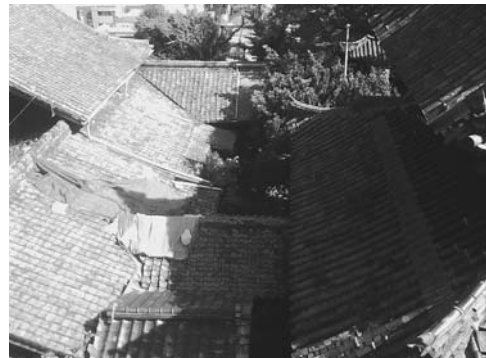
leaky roof detail
