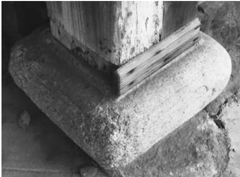
damaged pillar base
