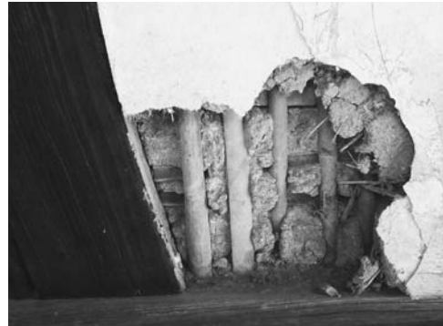
crumbling wall detail
